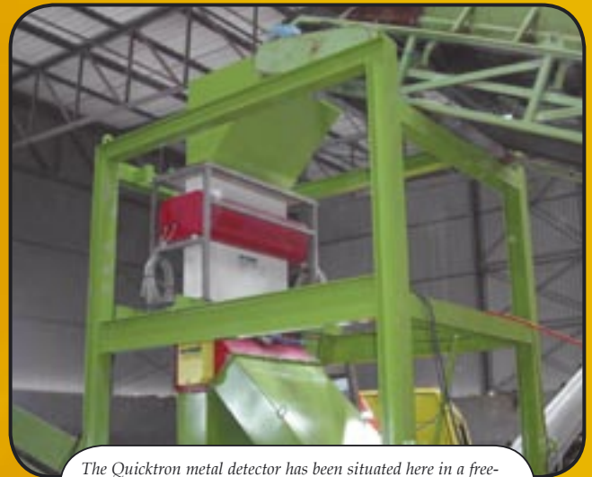
The Quicktron metal detector has been situated here in a free-fall line for the processing of demolition wood. This detector serves as an extra check before the wood is processed in the chipboard industry. This guarantees a product which is 100% metal-free. A top belt magnet first makes the wood completely iron-free. This prevents unnecessary switching of the flap and the associated product loss.
