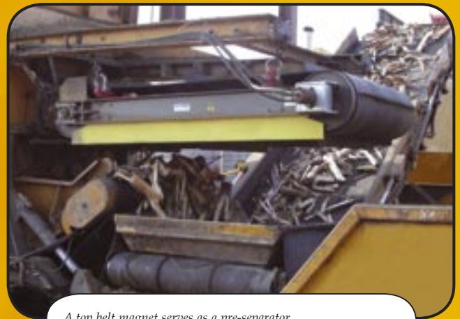
A top belt magnet serves as a pre-separator.
